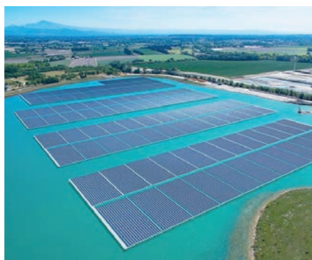
The largest photovoltaic plant in Europe floats on a lake in France. Over 46,000 panels supply about 4,700 households. Picture: ©Akuoenergy
